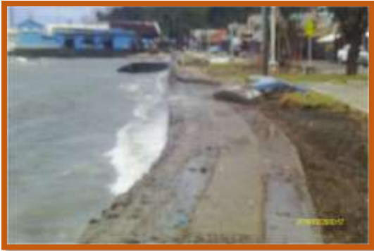
Seawall damaged - after TC Winston
