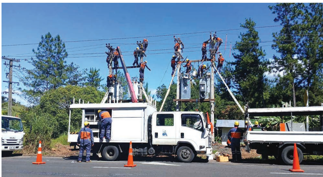
EFL Team installing Auto Boosters at Veisari to improve efficiency of power supply to its customers.
