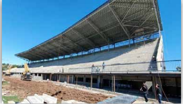
Govind Park project redevelopment - pavilion under construction. The pavilions at the Govind Park ground was completely damaged in 2016 by cyclone Winston.
