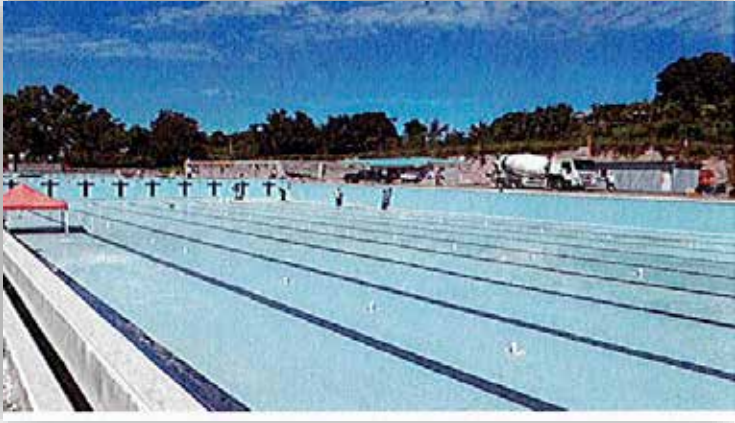
Lautoka main Swimming pool under construction at Botanical Garden. Three pools altogether were constructed, the main pool, warm up pool and children's pool.
