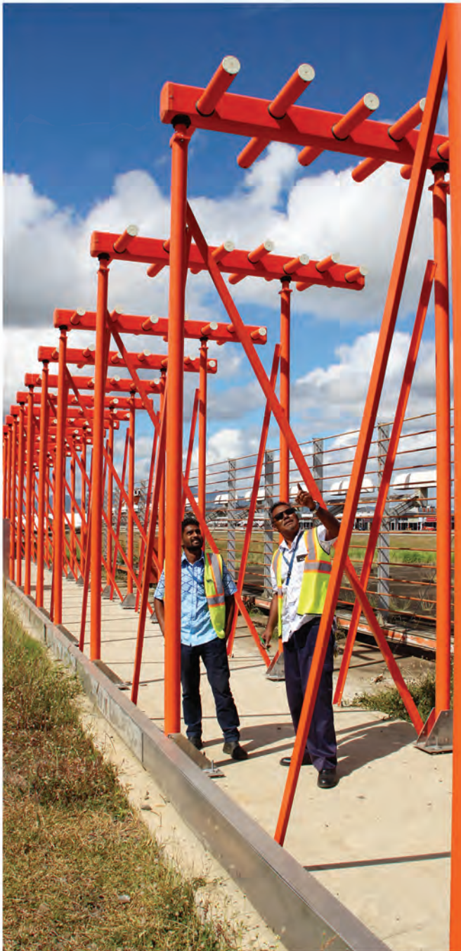
The new Instrument Landing System (ISL) Localiser at Nadi Airport.
