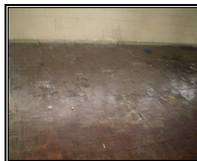
Room/Cube 4 damaged floor
