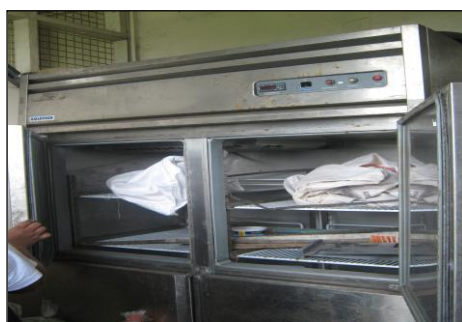
Cooler not working for more than 10 years
