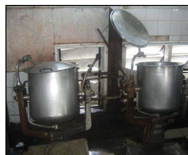
Steamers are very old and leaking
