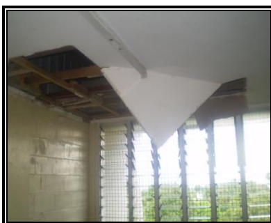
Room/Cube 4 damaged ceiling
