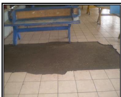
Broken tiles in dining hall
