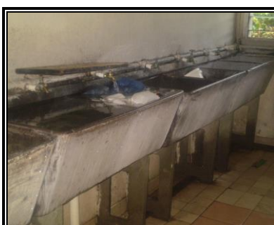
over flowing of water in the sink
