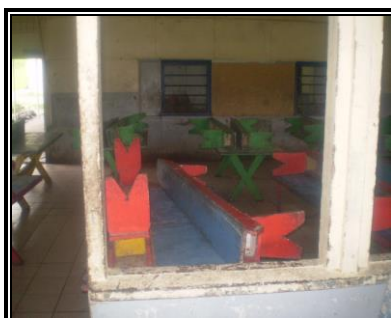
Poor state of dining room
