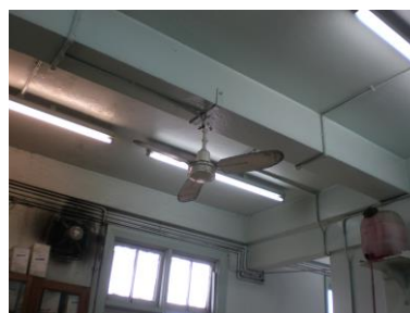
Faulty exhaust Fan in Mortuary
