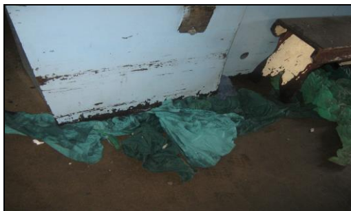
Clothes used to stop leakage from the laundry machine.
