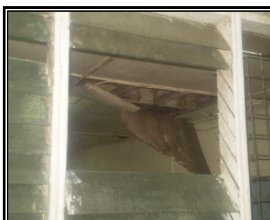
Broken louvers and ceiling
