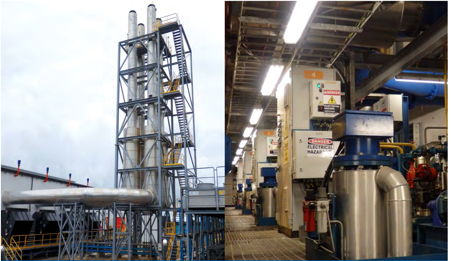
The above pictures show the newly constructed 35MW HFO Power Plant that was commissioned on the 14th November 2015. FEA spent around $70.3M on this project.
