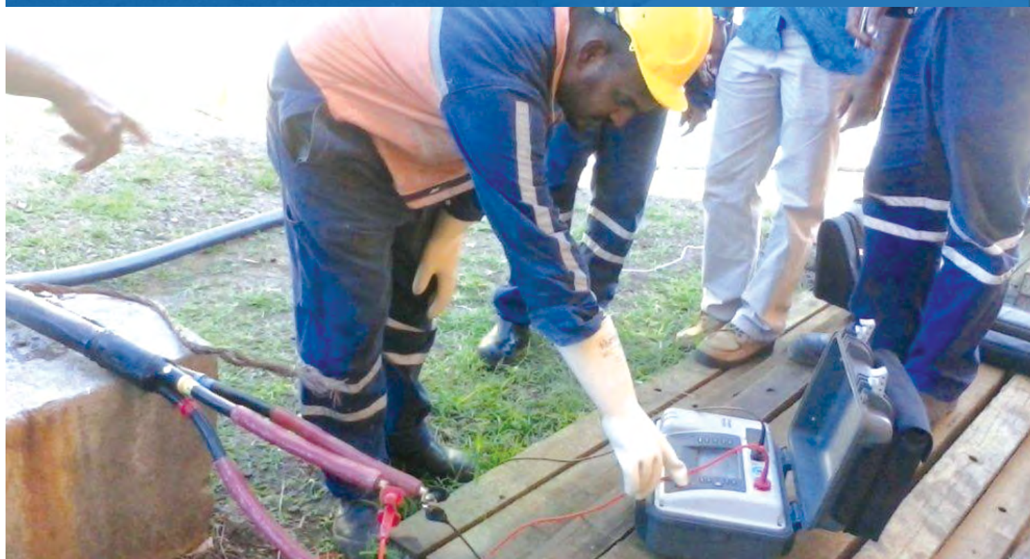
FEA employee carrying out the testing of new cables before being commissioned by the FEA technicians.
