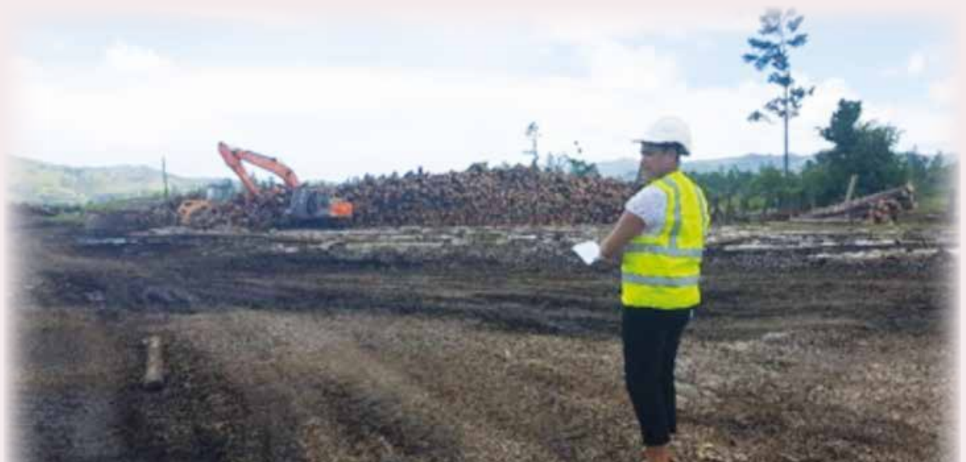
A FCC Officer conducting site visit at the Tropik Wood Mill in Drasa, Lautoka.
