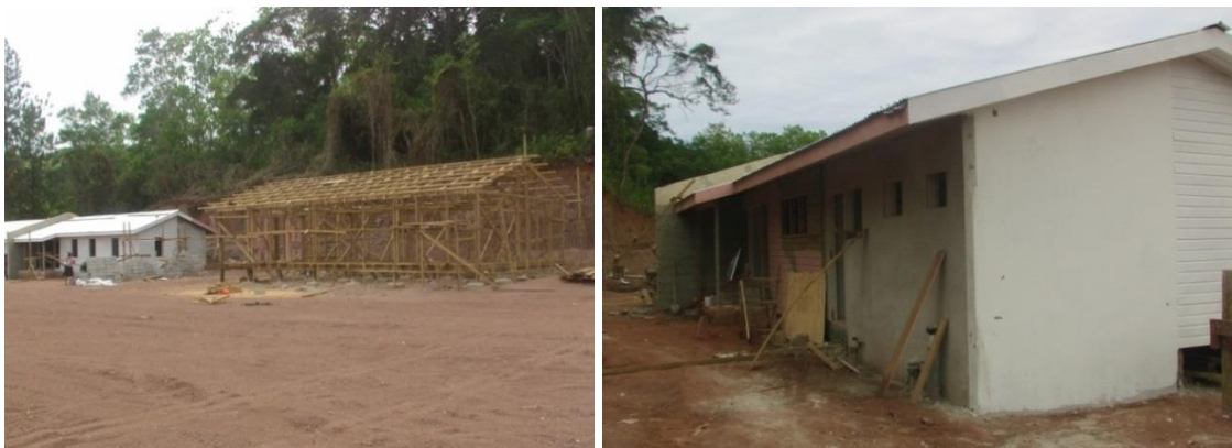
Figure 18.7.1: The audit site visit verification on the completion date, 11 th December 2015 reveal that the Kubulau Duplex quarters were still in progress.
