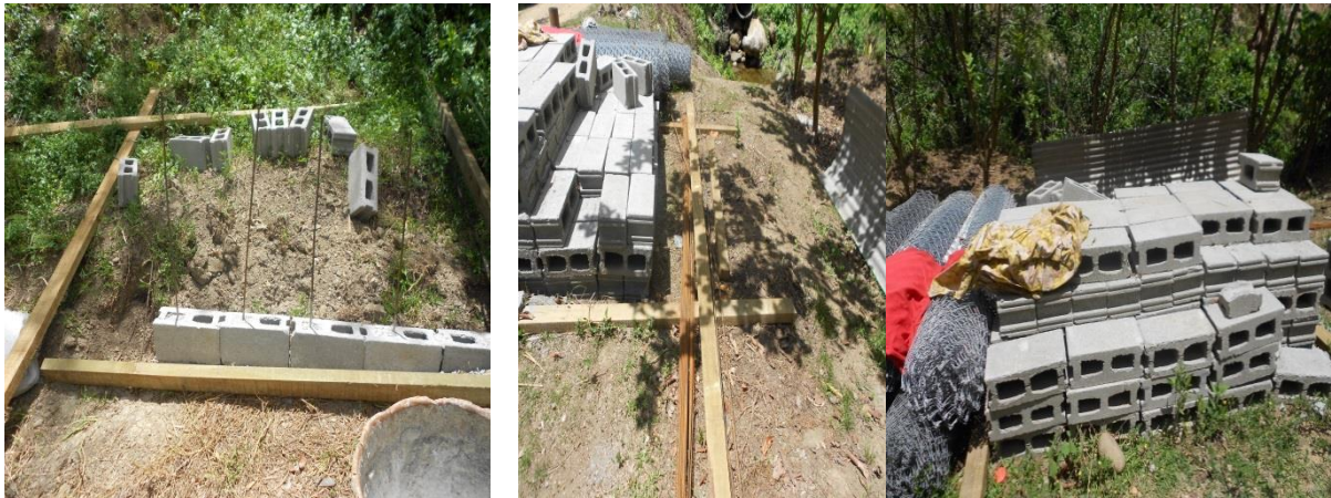
Figure 18.5.1: – Poultry Farming Project (Korolevu Village, Navosa).Materials has been lying idle as at the date of the audit site visit verification on 19/11/15.
